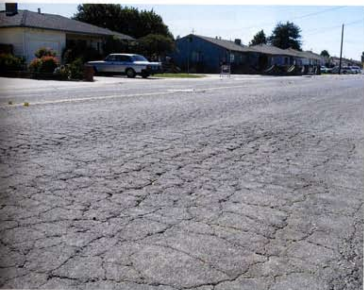
Pavement condition before AR/PMAR (asphalt-rubber/polymer modified asphalt-rubber) three-layer cape seal in Watsonville, Calif.
